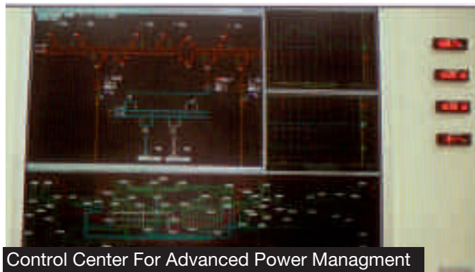
Power Plant Deir Aamar
