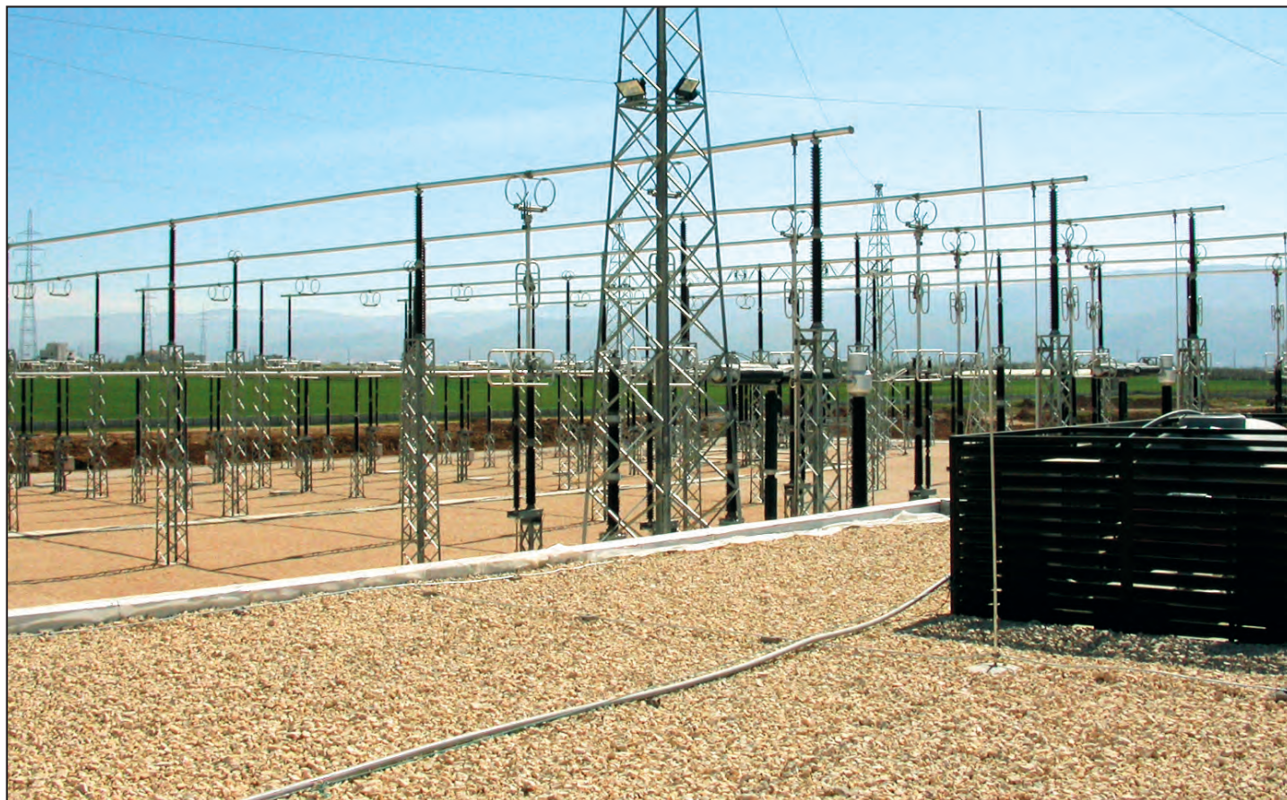
Seven countries interconnection network (400 KV)
