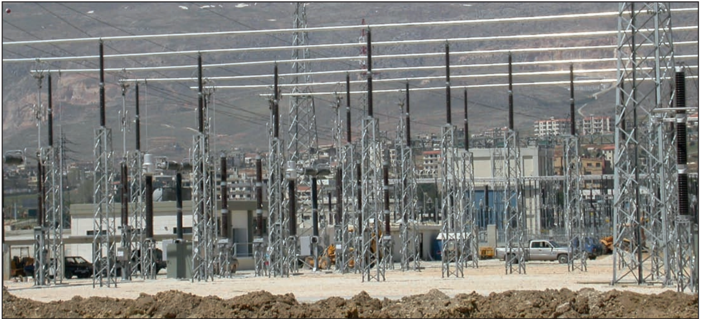
400 KV Interconnection network between several arab countries in Ksara.
