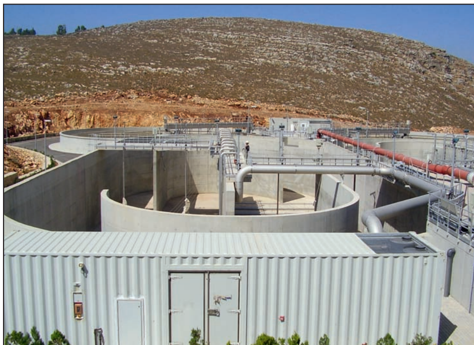
Wastewater treatment plant in Nabatieh
