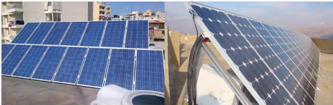
Figure 3: two PV projects installed by CEDRO
