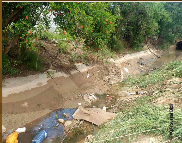
Figure 3: A heavily deteriorated canal section
