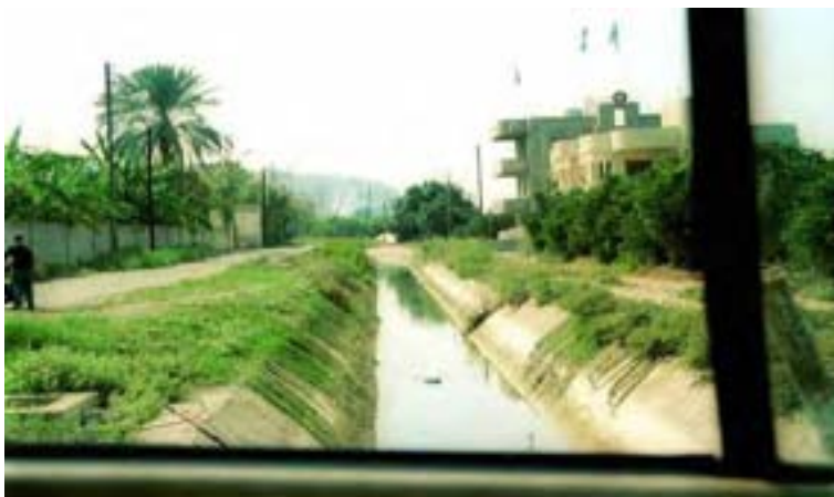
Photo 46: Irrigation channel, Sarafand (Litani project)
