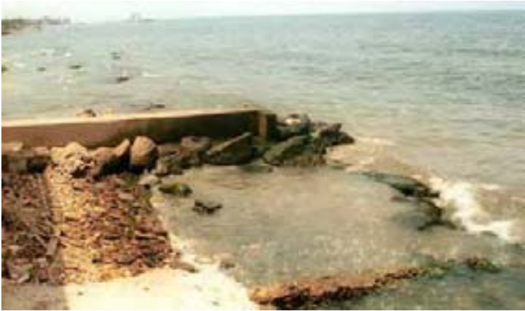
Photo 52: Main wastewater outlet in Sarafand
