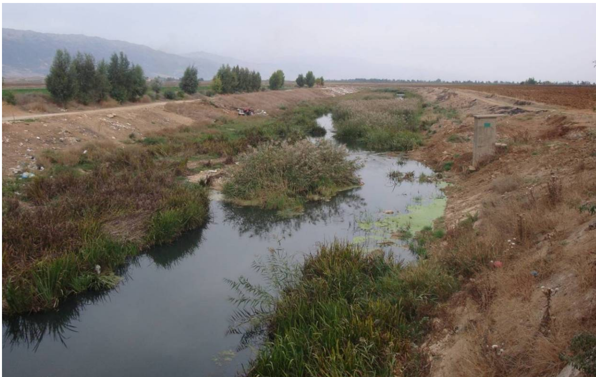
Photograph 7.1: Over-excavated Litani riverbed in Joub Jenine: vegetation development and sedimentation are recreating a smaller and meandering riverbed
