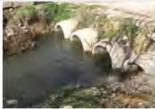
Culvert for the Access to the Farm (4 pipes D=1200)
