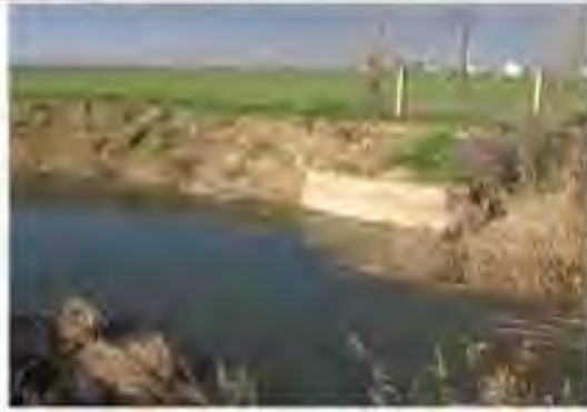
Old Culvert Destroyed
